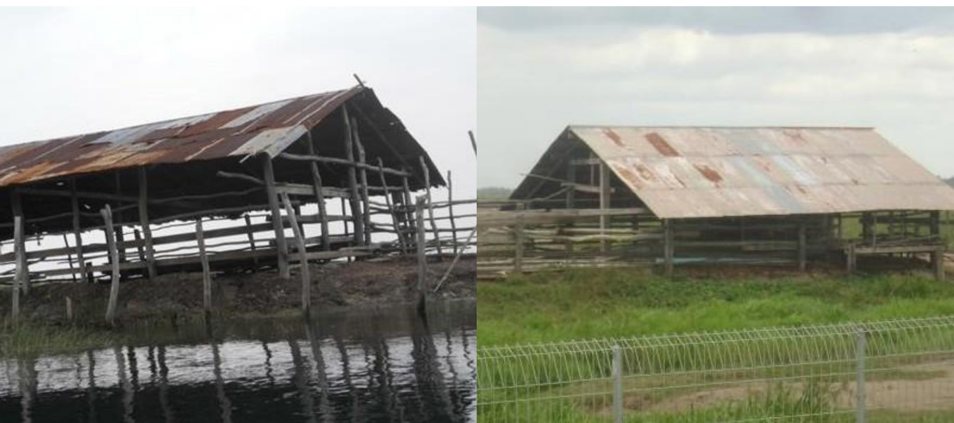
Figure 37 Pen with roof
